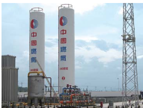
Left: Construction site of mid-range pressure natural gas network in Wuhu Right: Liquefied Natural Gas (LNG) tanks
